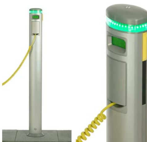
Figure 28: On-street electric vehicle charge point 71
